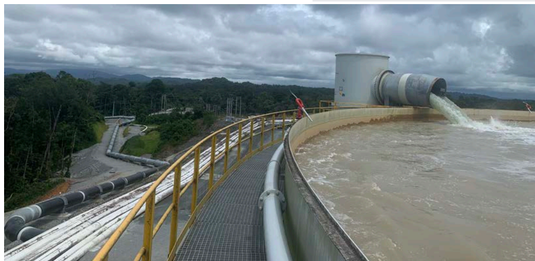
Decant Water Commissioning
