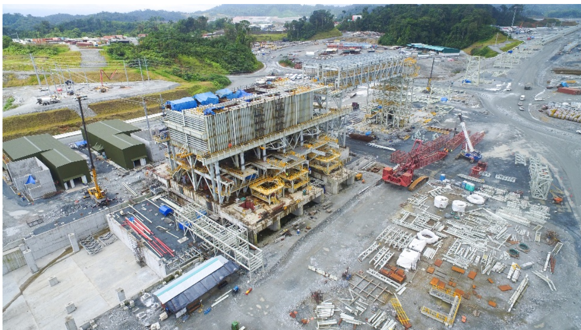
Secondary/Pebble Crushing & Overland Conveying
