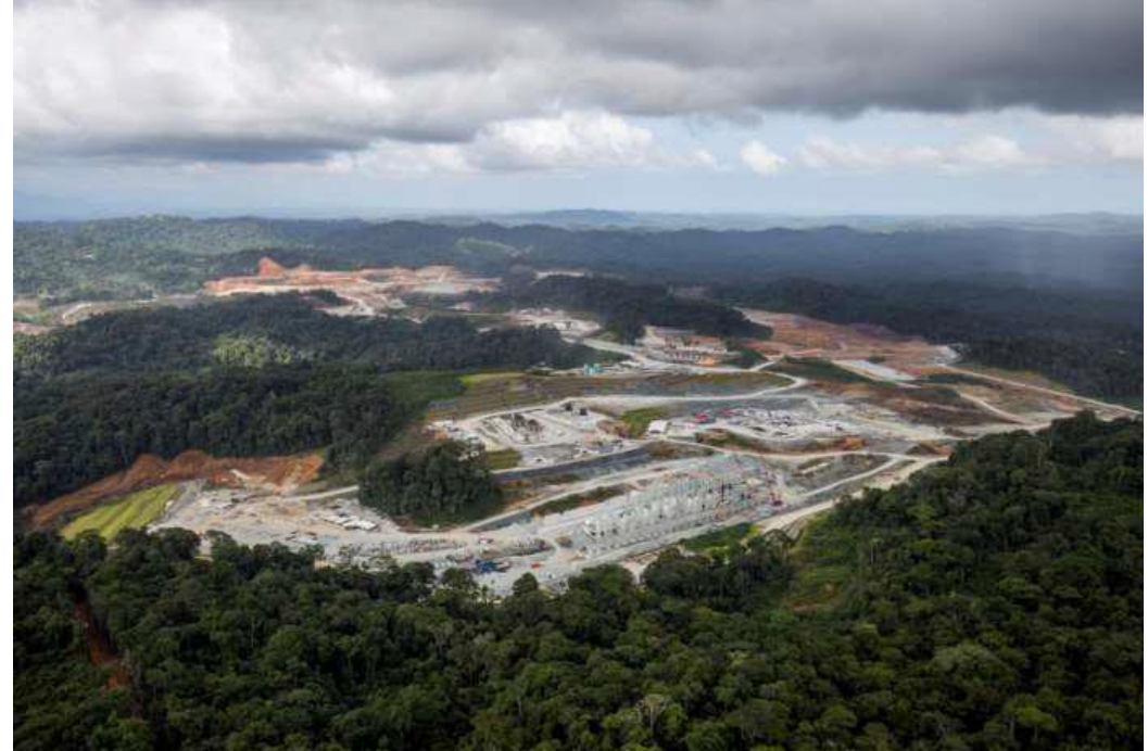
PROCESS PLANT OVERVIEW 01-FEB-2016
