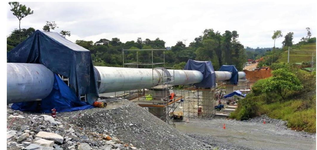
Process water pipeline
