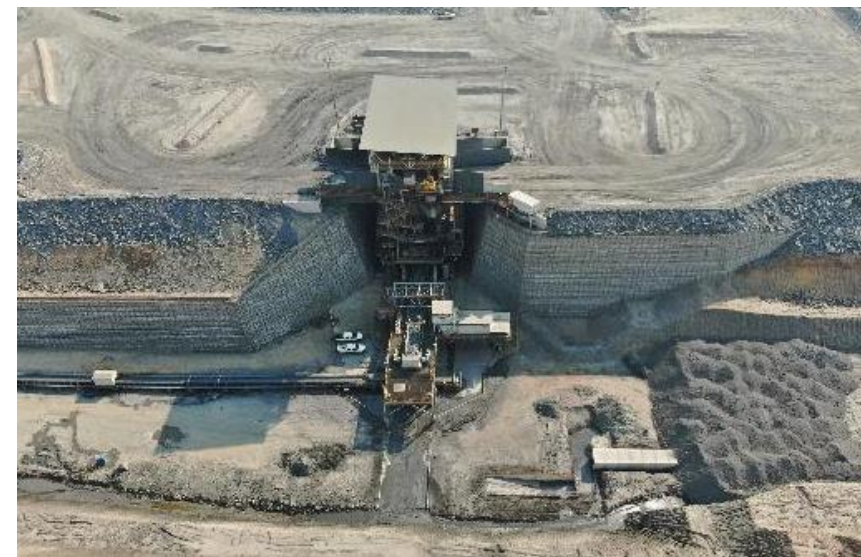
In Pit Crusher in Stage 3
