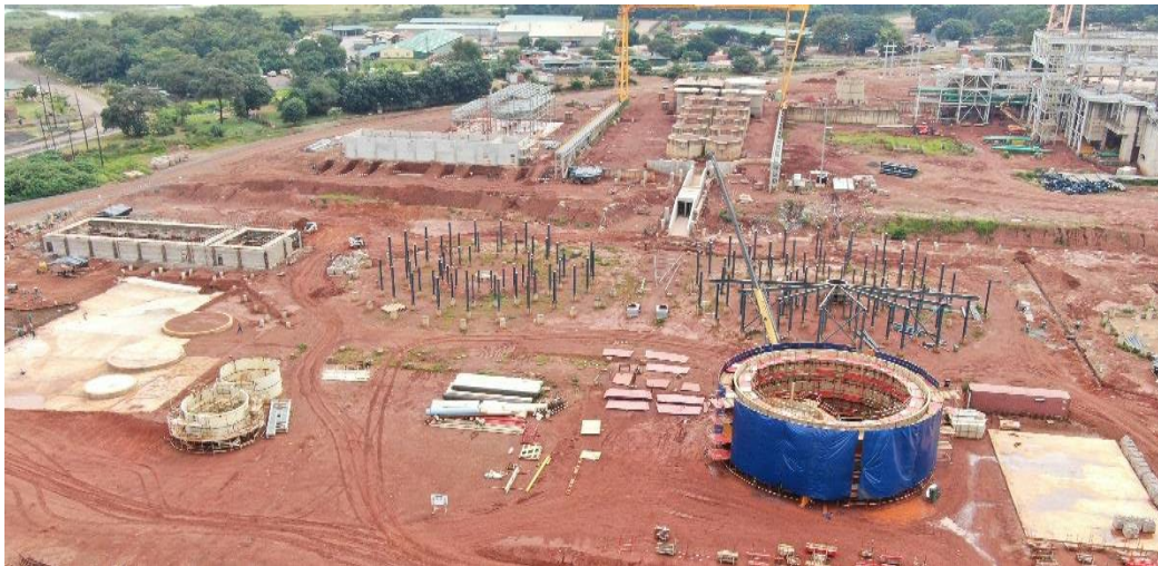
Rougher flotation area, newly installed over head crane
