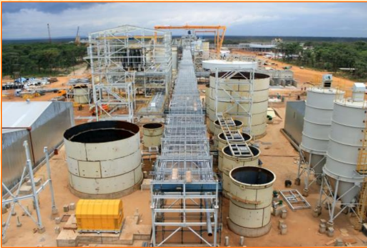
REAGENTS, DEPRESSANTS AREA & PIPERACK LINE 31-DEC-2013
