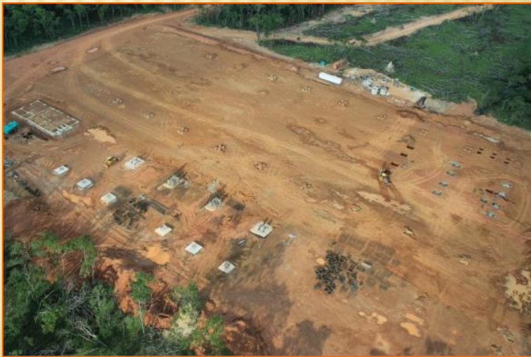
ABB SWITCHYARD 30-DEC-2013
