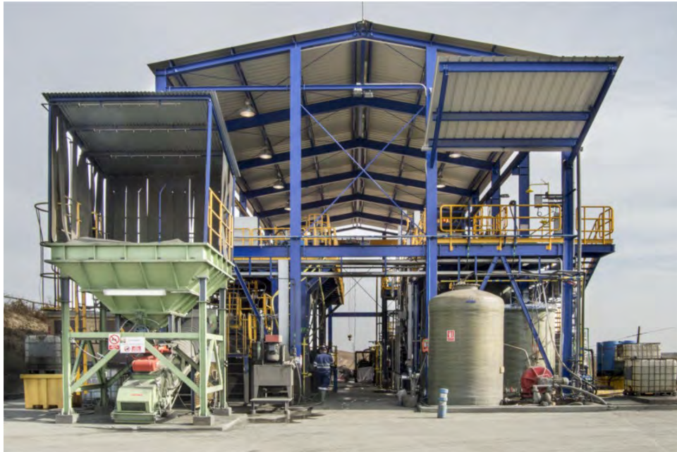
Figure 13-2 2 Pilot Plant Front View
